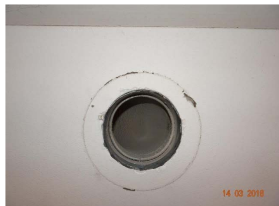
Abbildung 195: WNG ID 820: ABL-Rohr, Bad
