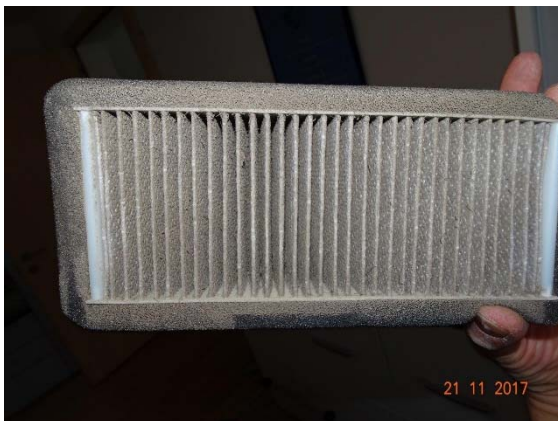
Abbildung 30: WNG ID 120: Zuluftfilter
