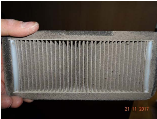
Abbildung 21: WNG ID 110: Zuluftfilter
