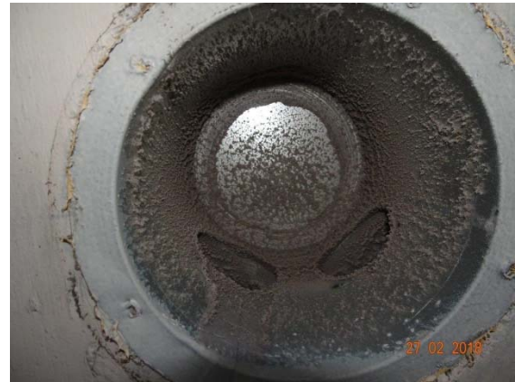
Abbildung 161: WNG ID 720: ABL-Rohr, Bad
