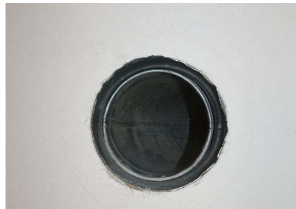
Abbildung 202: WNG ID 820: ABL-Rohr, Bad
