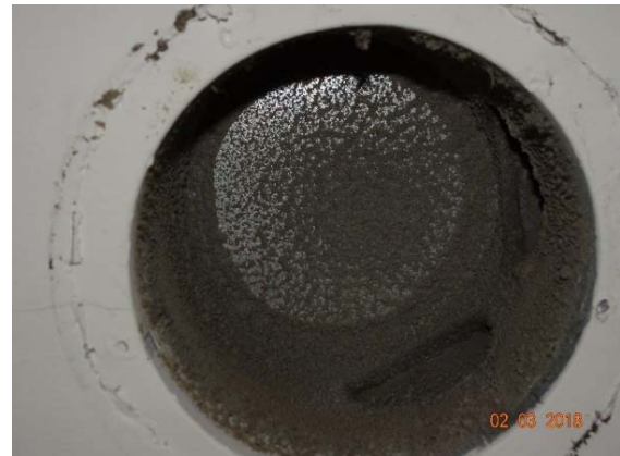
Abbildung 170: WNG ID 730: ABL-Rohr, Bad
