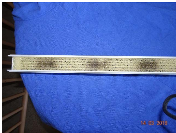
Abbildung 185: WNG ID 810: Zuluftfilter.
